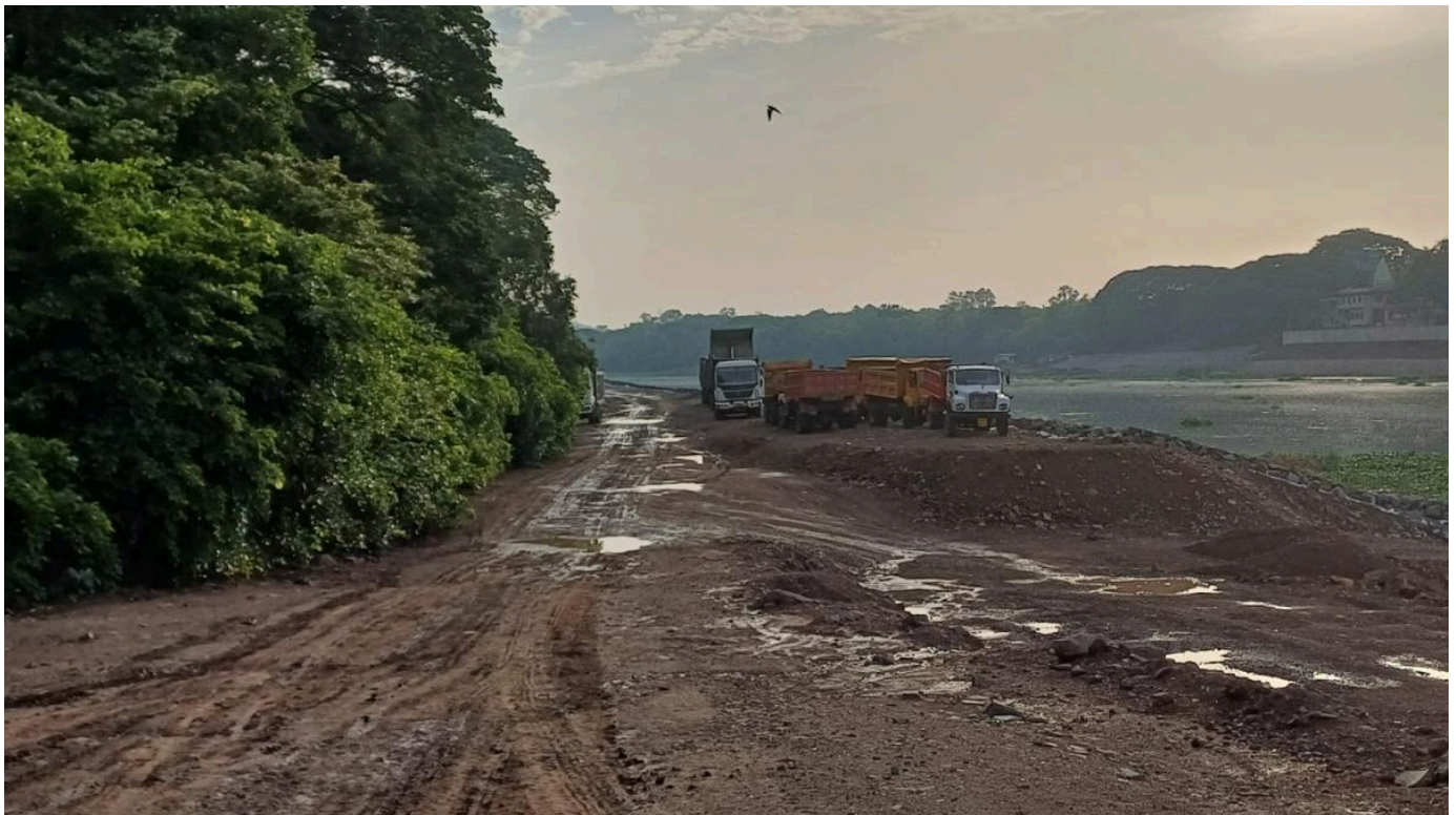
Construction activities along the banks of the Mula Mutha (Image Source: Jeevitnadi)
